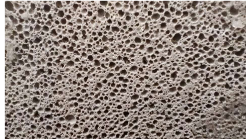
Sawn cross section of a typical RAAC panel (Loughborough University)
